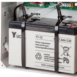
Battery restraining ties
